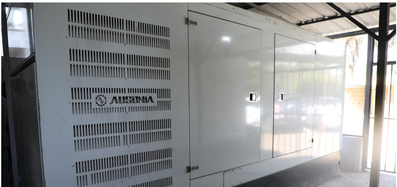
The Data Center
